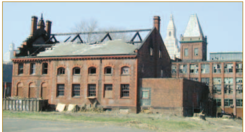
View of former Capewell Horse Nail Company administration building on Governor Street, showing fire-damaged roof.
